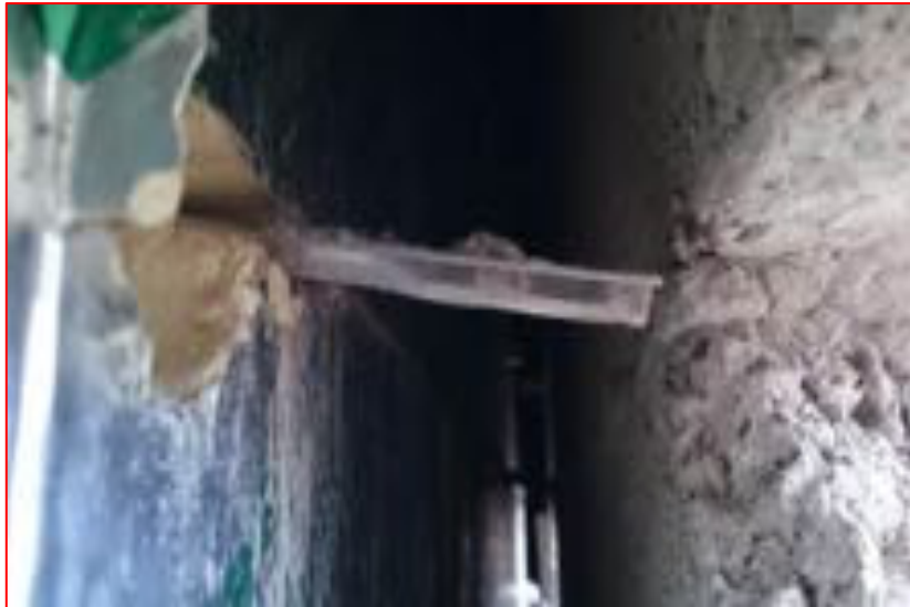
Image 8: Photograph from the survey reports showing the lack of embedment. This is an example of no embedment of a wall tie at Howdenhall Centre.
