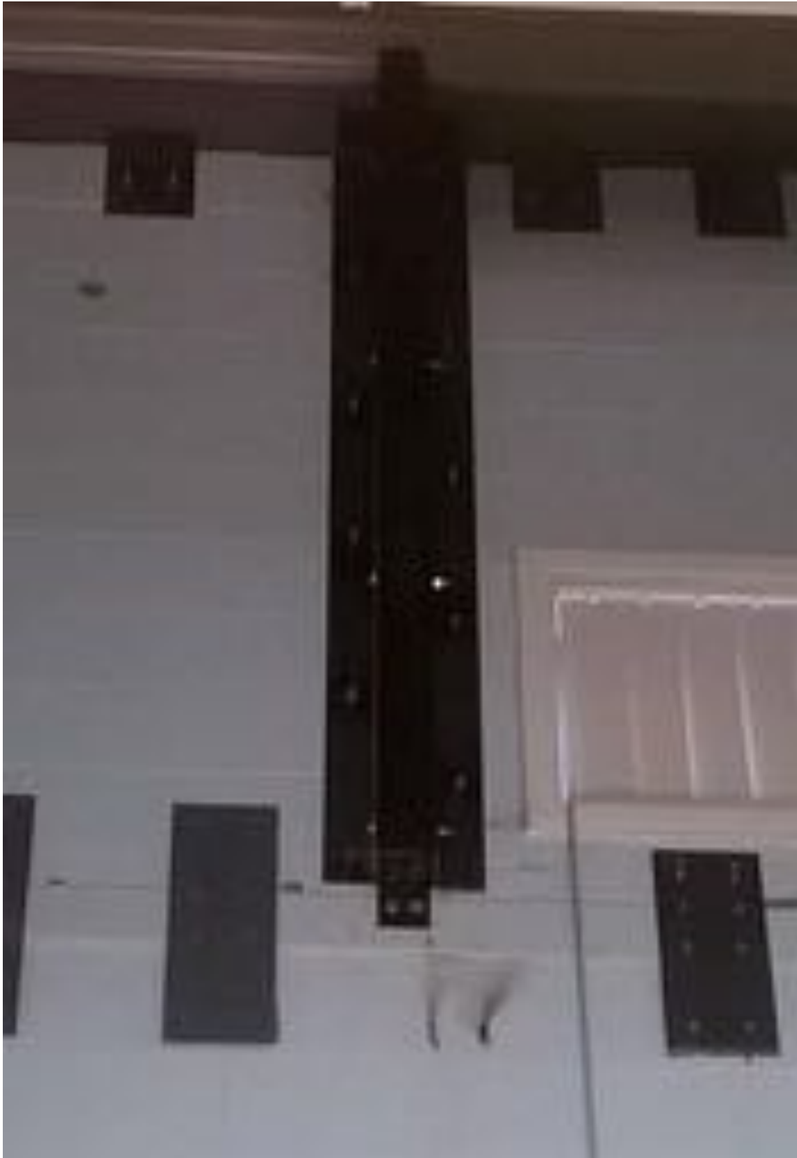
Image 18: Vertical windpost spanning from intermediate horizontal beam to roof beam and wall head restraints fitted to both beams as installed prior to boxing in and painting at Oxfangs School.
