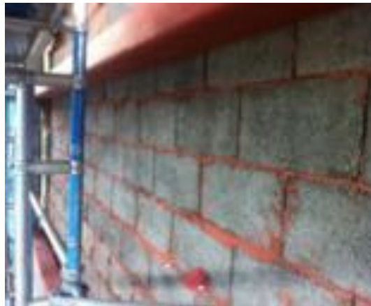
Image 30: St Ninian's High School; "No wall ties have been installed into a large section of the wall."
