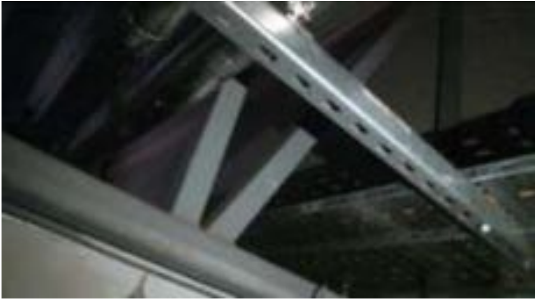
Image 21: Example of a breach of fire compartmentation from fire-stopping survey of Oxfangs School, dated 22 nd August 2016: "there is no plasterboard above the fire door, therefore creating a large breach in the compartment. the area is not fire stopped and a breach exists."
