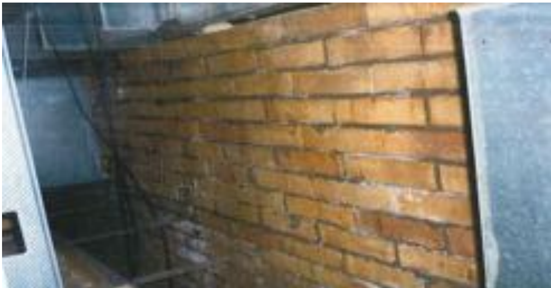
Image 27: Photograph from Duncanrig Secondary School. 'Note no ties or head restraints to inner face of outer brick leaf'.
