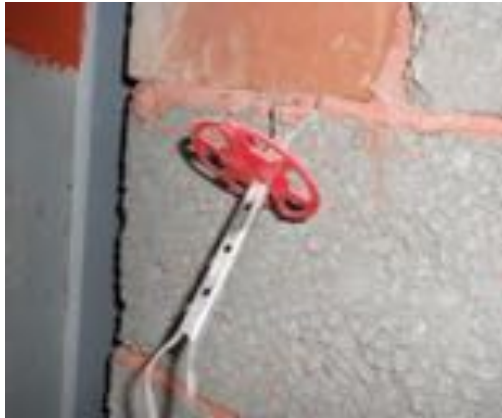
Image 29: St Ninian's High School; "Photo showing one of the defective wall ties (no embedment) in place behind the internal skin of blockwork in the sports hall."
