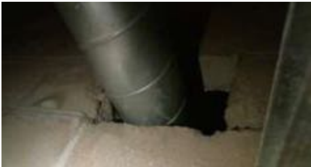
Image 22: Example of a breach of fire compartmentation from the fire-stopping survey of Royal High School, dated 22 nd August 2016 : "the pipe has not been fire stopped and a breach exists."
