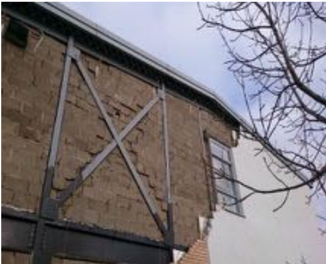
Image 5: Photograph of exposed inner blockwork leaf of gable after removal of insulation demonstrating the recessed blockwork in the braced bay which resulted in extending the width of the cavity.
