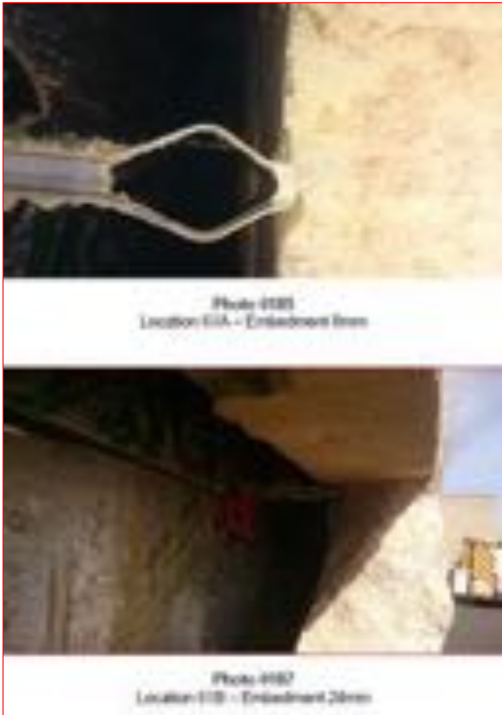
Images 6 and 7: Photographs from survey reports showing the lack of embedment. These are two examples from Craigmount High School, showing embedment of 0mm and embedment of 24mm.
