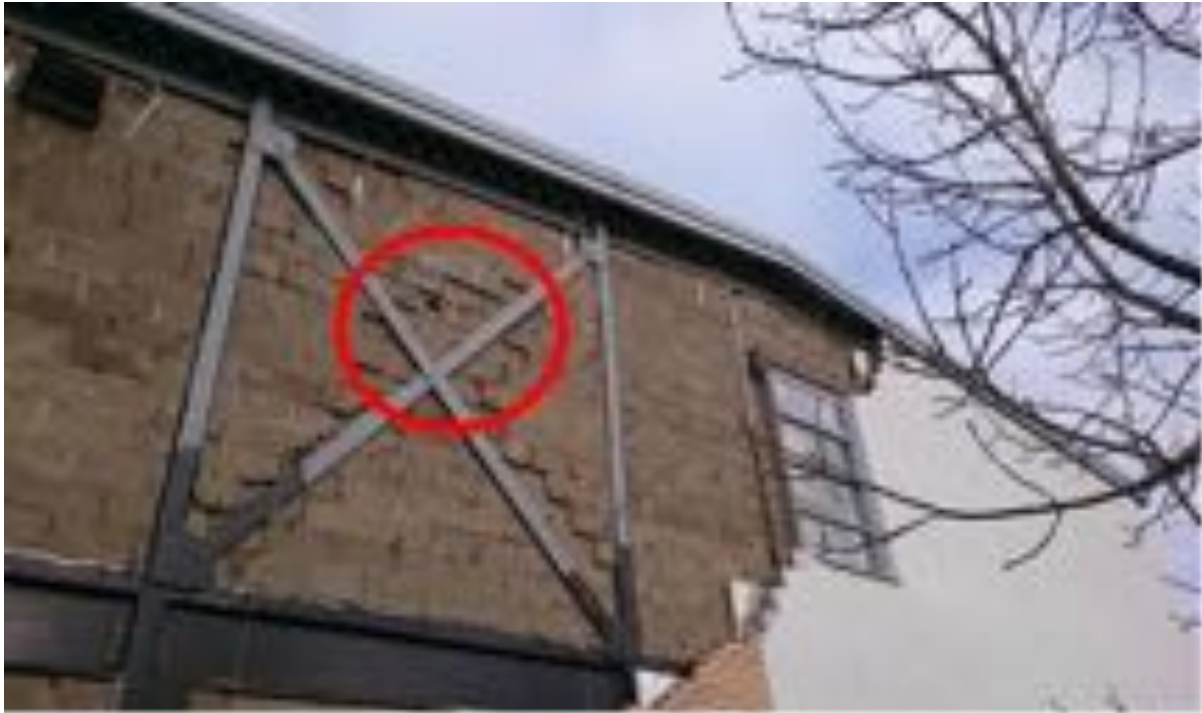
Image 23: Photograph of the collapsed section of the Oxgangs gable wall.
