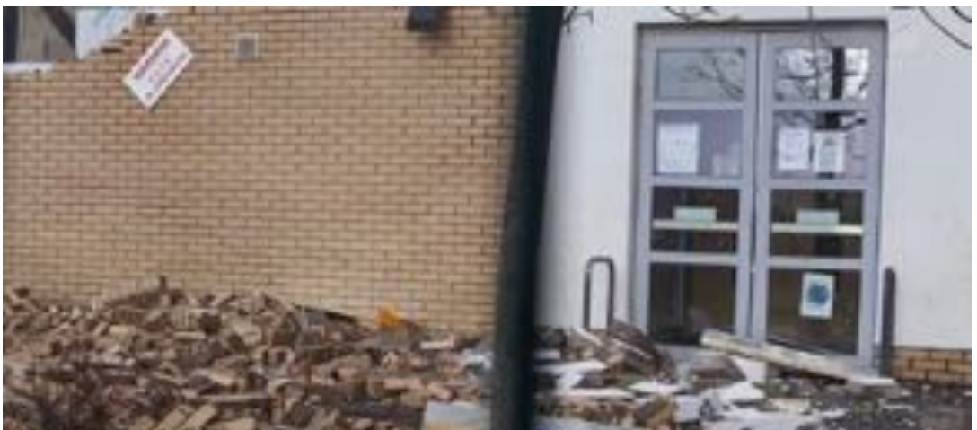
Image 4: Photograph taken at Oxfangs School of the gable wall after the collapse.
