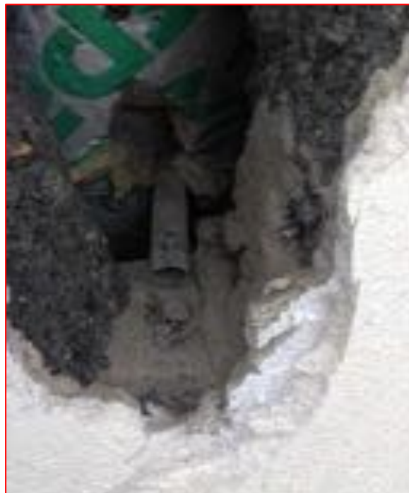
Image 9: Photograph from the survey reports. This photograph shows very limited embedment of a wall tie at Forthview Primary School.
