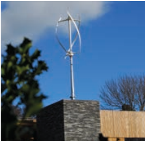
The quietrevolution wind turbine on top of the John Hope Gateway, RBGE.
